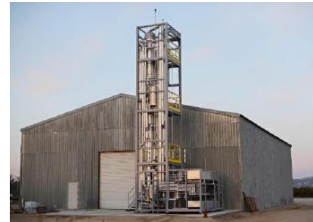
Customer Installation Coleambaly, NSW Australia
