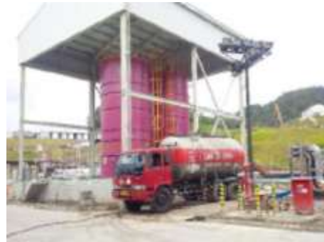
Load acid for ph Control
